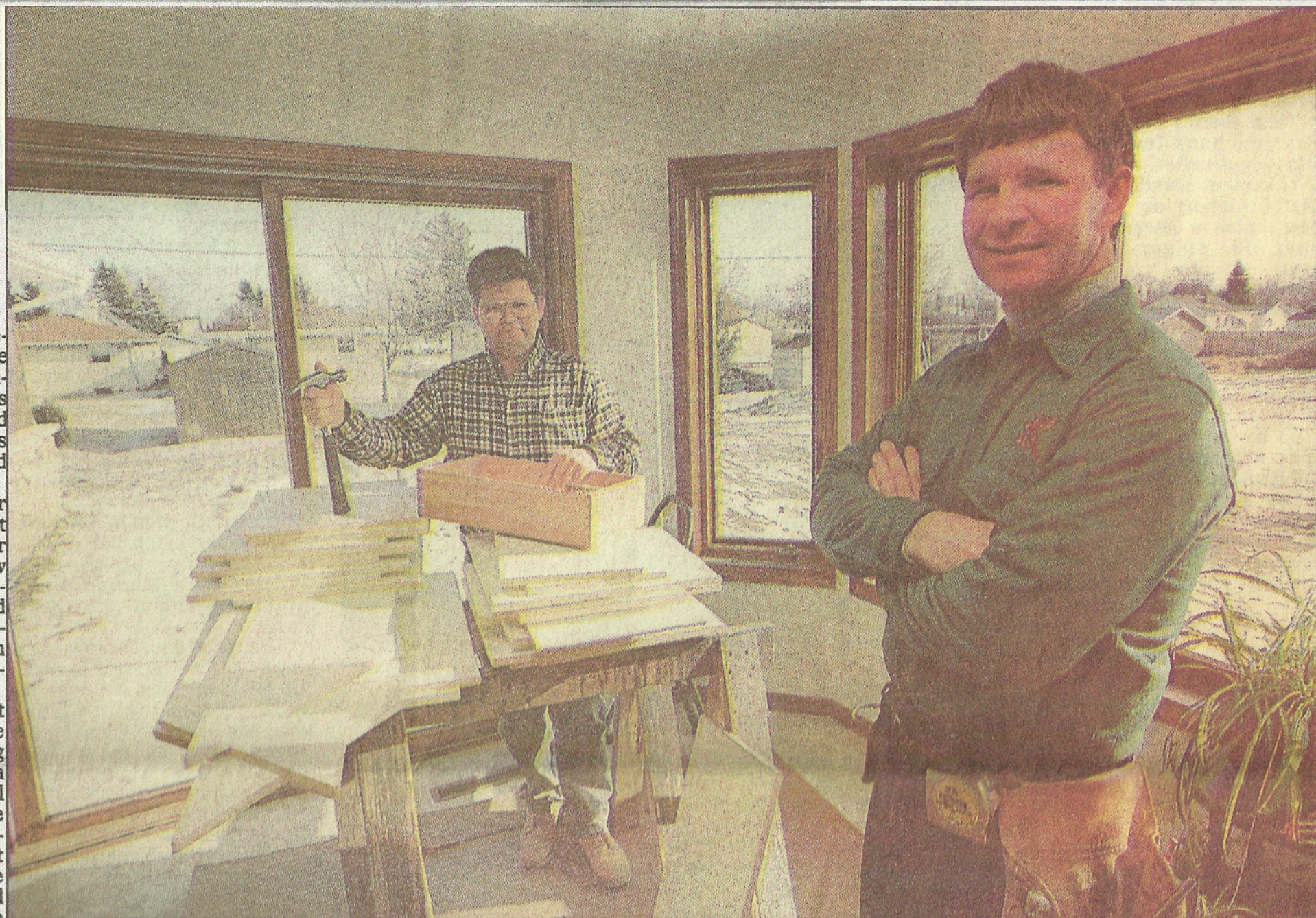
BROTHERS AND BUILDERS: Steve Leonhard, left, and his brother Cletus at work in the dining area of a home they have been working
