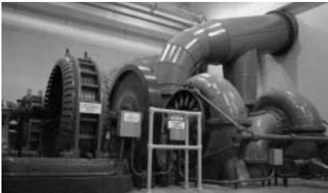
NORTH AMERICAN HYDRO, INC.
